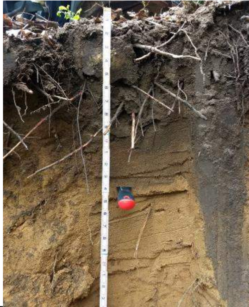
Photo 1: TP6 Upper Side Wall Looking Southeast
